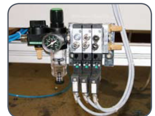
Pneumatic unit with filter and self-governing relay.
